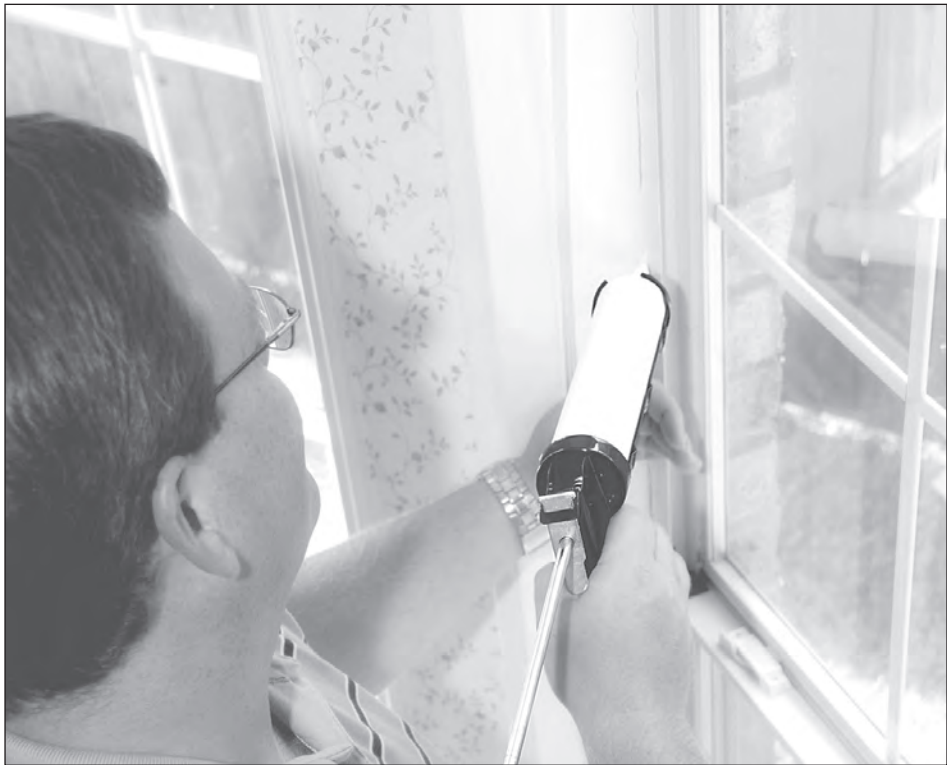
Leaks around windows and doors can prove costly if they're not addressed promptly. As winter approaches, investigating for leaks and addressing any that are found can save money and ensure a home stays comfortable when the temperatures drop.
