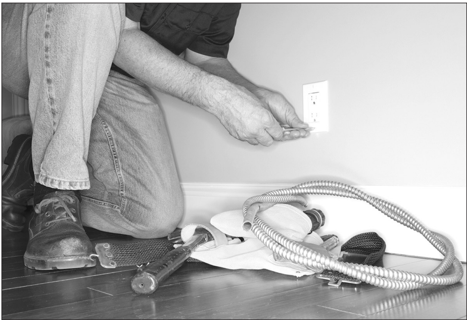
Contributed photo When cleaning a home, homeowners can pull double duty and look for potentially hazardous electrical issues that could be dangerous.
